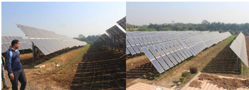
1 MW Agri Voltaic Solar Power Generation Plant, was installed in Village: Amrol, Ta. Anklav, Dist. Anand, Gujarat by Anand Agricultural University in collaboration with Gujarat Industries Power Company Limited
