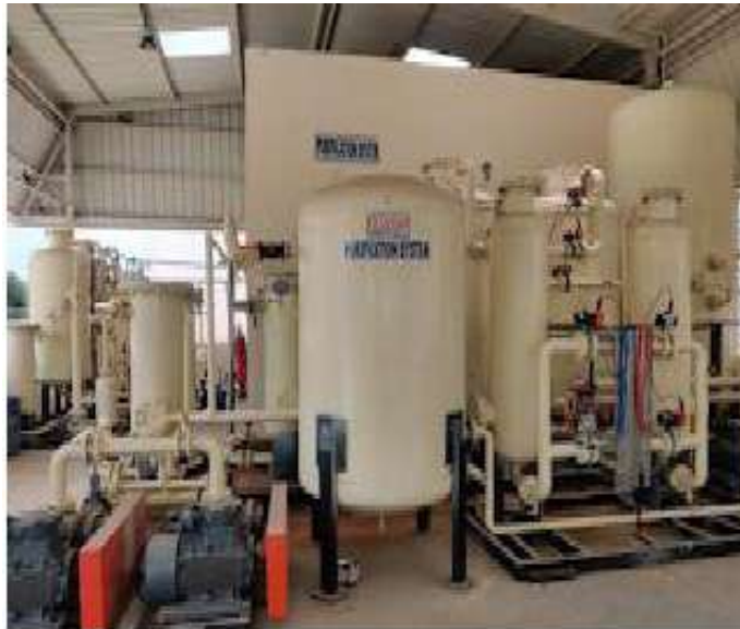
Fig.13: VPSA Purification System
