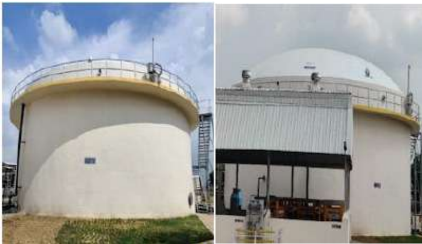
Fig.11: Fixed Dome type Biogas Digester and Gas Holder
